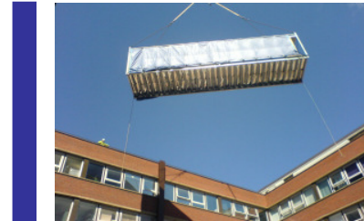
Top: One of fourteen modular steel cleanroom frames is lifted carefully over a six-story hospital wing.
