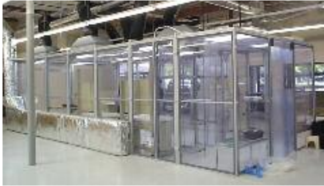
Rather than ceiling plenums and air chases in the walls, this room uses an elaborate system of ducting to recirculate air leaving the room, and bringing it back in through the ceiling to pass through the HEPA filters before re-entering the room. The gowning area on the right end of the room provides technicians a place to gown before entering the main cleanroom, reducing the risk of contamination.
