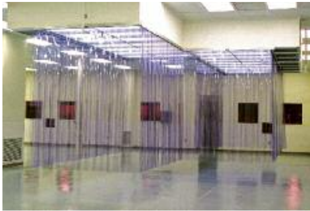
This enclosure is in As Built state, before equipment and materials are moved in. Notice that it is within an existing room and takes advantage of the air conditioning infrastructure that is already installed. Cleanrooms are certified by the manufacturer in an As Built state.
