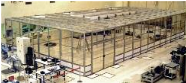
Modular cleanrooms as large as 5,000 square feet, and even larger, are often required for assembly lines, packaging operations and other environments.
